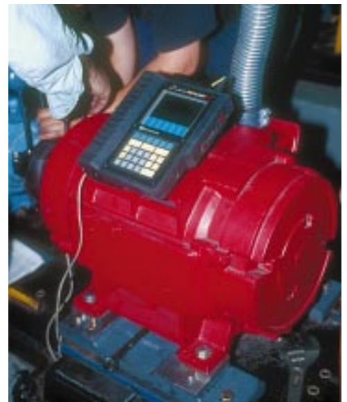
When alignment is completed pump and motor are typically aligned to .003".
