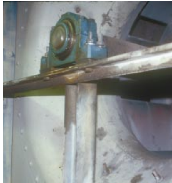
New SAF Pillow Block Bearings, bracing, and alignment.
